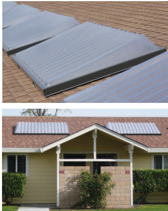
Fig. 2. For this project at a mid-rise apartment building in Sacramento, California, Harpiris installed 65 collectors across 35 separate systems, ranging from one or two collector systems pre-heating individual tankless gas water heaters, to up to eight collector arrays pre-heating pairs of 100 gallon water heaters. Federal and utility incentives paid for more than 60% of the total system cost. (Top) Eight SunCache collectors in parallel, feeding 200 gallon storage. (Bottom) Individual collectors installed on individual units with tankless water heaters. Photos from Harpiris Energy
