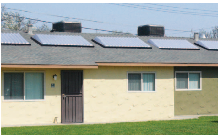
Fig. 11. Forty SunCache collectors were installed in three separate systems at an apartment complex in Hanford, California. Each system uses parallel pre-heating arrays ranging from 11 to 15 collectors, pre-heating pairs of high efficiency commercial gas water heaters. The entire project took less than 100 man-hours to install. Photo from Harpiris Energy
