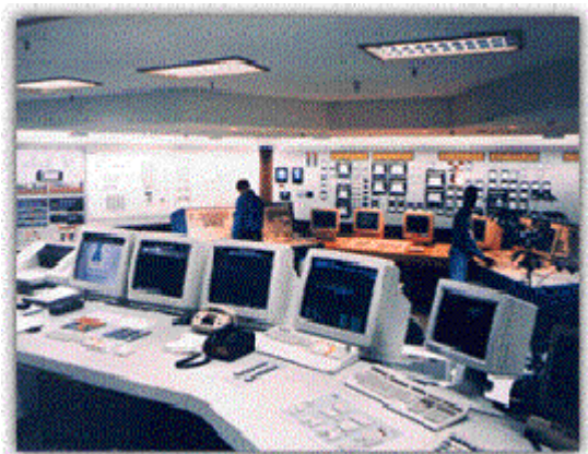
Fossil Fueled Power Plant Control Room STN ATLAS Elektronik GmbH
