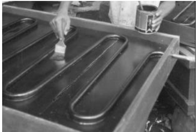
After the red lead paint or primer, paint the topside of the absorber with two layers of dull blackboard paint.
