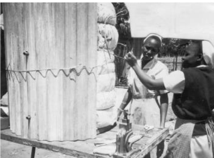
After surrounding the storage tank with insulating covers, entwine the covers with ropes or iron wire.
