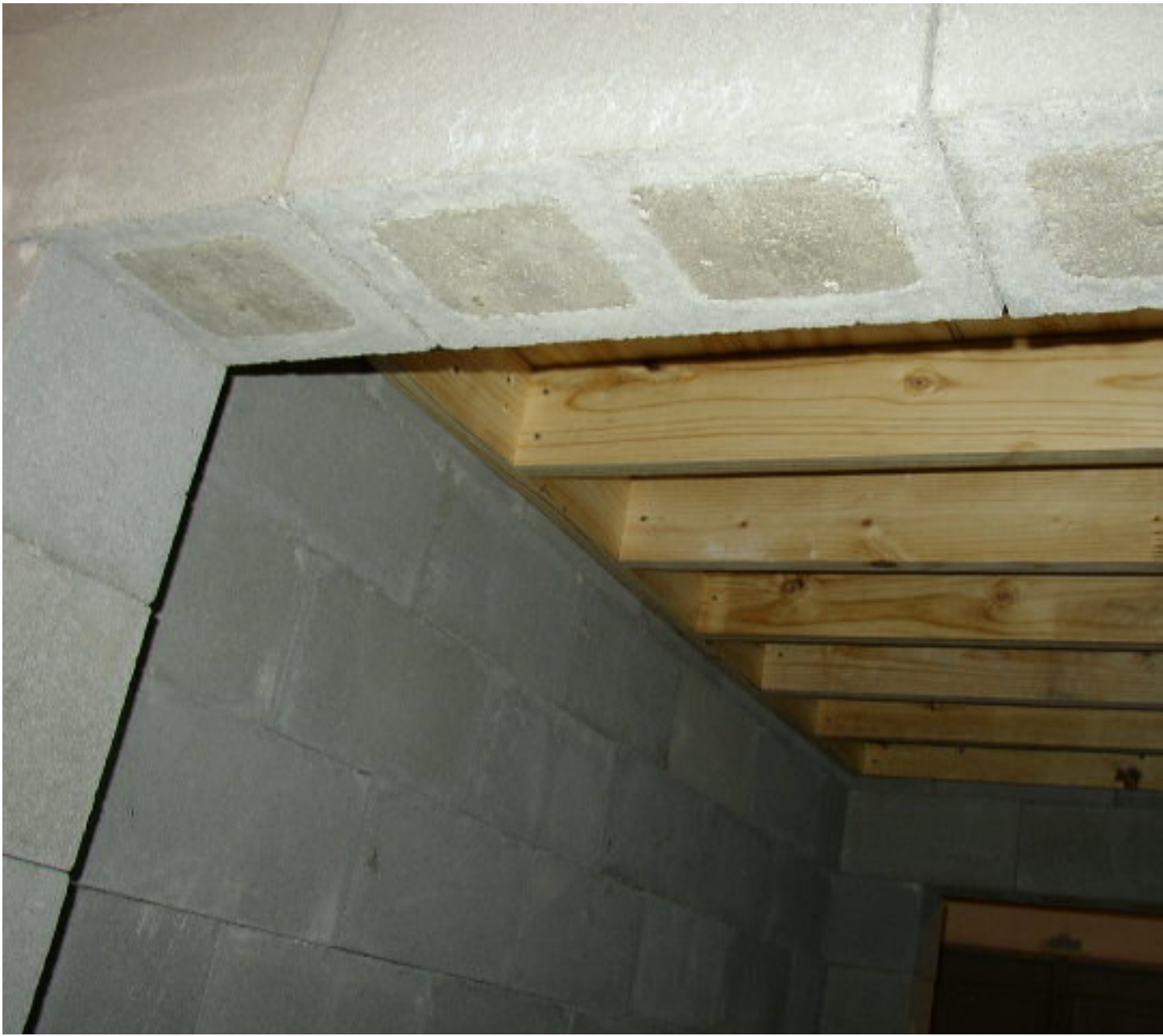
This is what the attic looked like before I poured the concrete:
